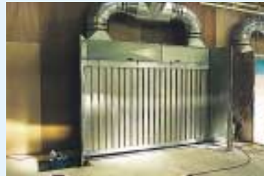
Spray booth with replaceable baffle plates for linseed oil painting.
