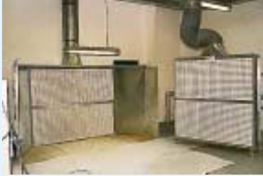
Spray booth with exhaust wall for painting of kitchen elements.
