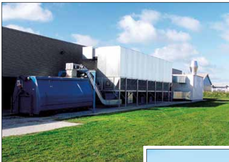
Aagaard chain filter at Danish furniture joinery with heat exchanger for return of air to the factory and with an Aagaard chip conveyor system for the transport of wood chips to a container.
